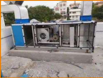
Air Handling Unit Services
