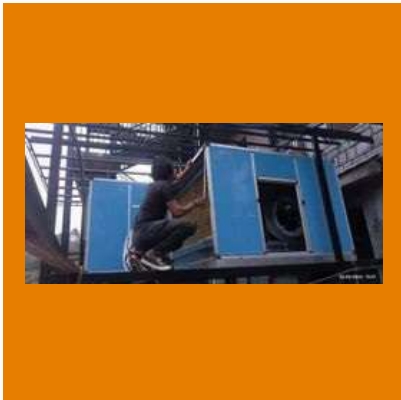
Air Handling Unit Installation Service
